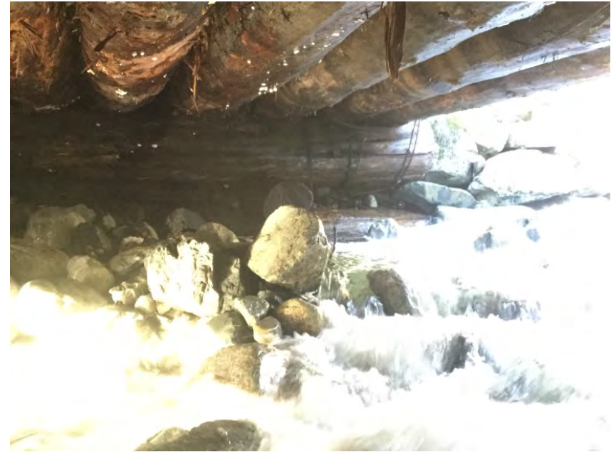
Scour noted upstream right bank
