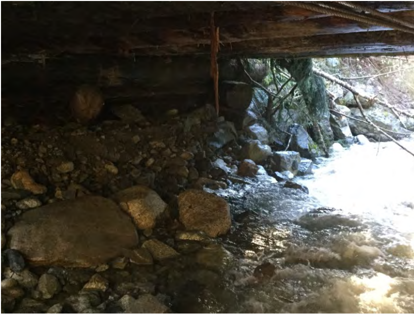
Scour noted downstream left bank
